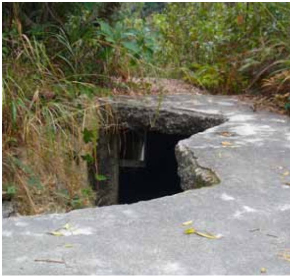
Figure 9: Blasted tunnel cover, Shing Mun Redoubt
