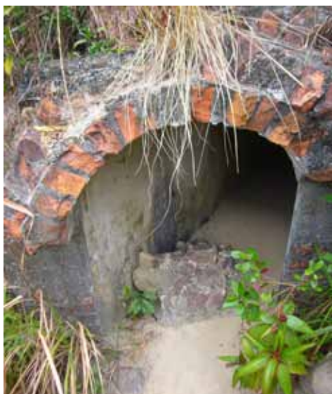
Figure 13b: Ruinous entry to the site of PB403, Shing Mun Redoubt Location F in Map 2. A number of tunnel entrances showed a brick vaulted lined construction method. This one connects to a PB403. Refer location F Map 2.
