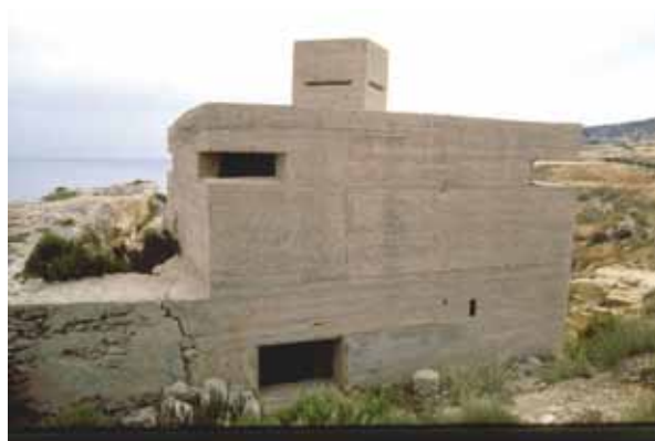
Figure 6: Another pillbox on Marfa Ridge but dating from WW2. It is likely that its concrete sides were painted with a camouflage pattern to resemble that in photo GDL 5. The large opening at its base may be an emergency exit.
